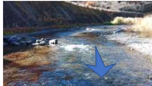
(b) Super dikes of assembled boulders installed in Kanna river, Gunma Pref.
